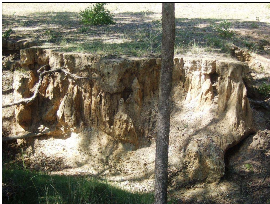
Plate 2: Erosion along drainage line.
